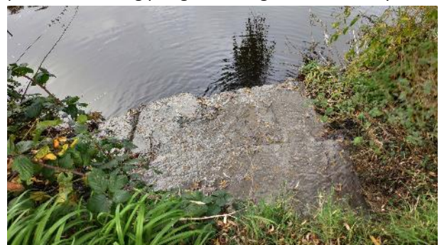
Plate 8.8 Significant pollution point source emanating from an unnamed, culverted stream along the Arklow river walk (November 2021)
