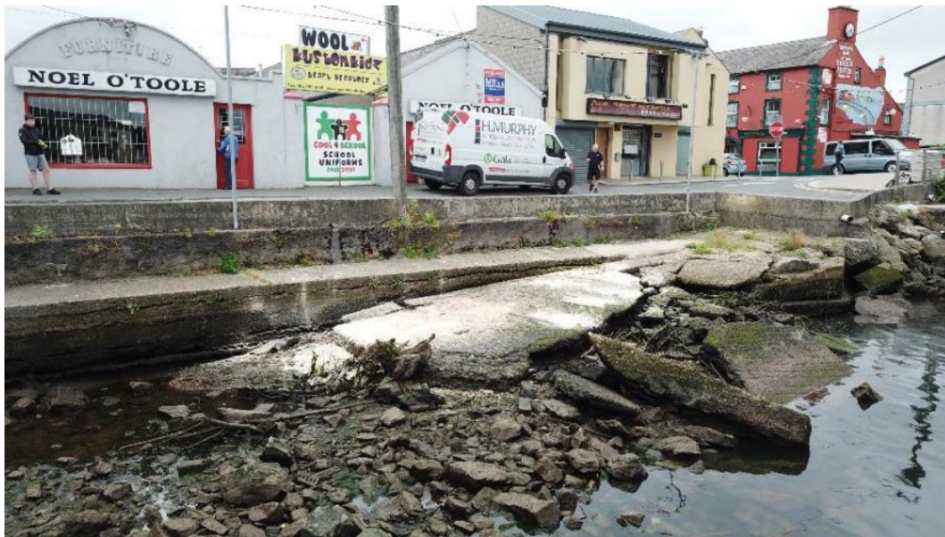
Figure 7.3: Slip at West End of South Quay
