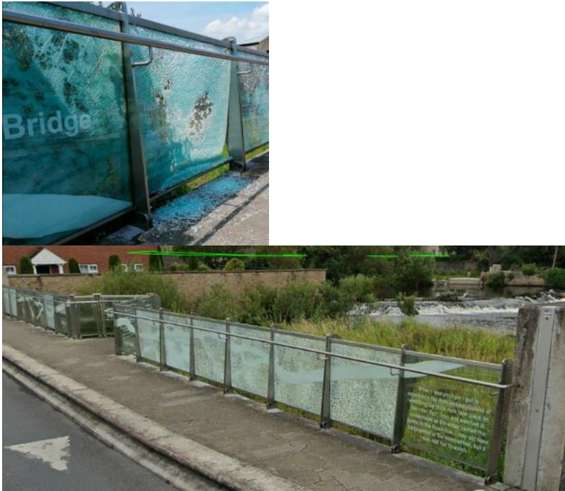
Figure 6.1: Photos of Damaged Glass Panels – Clonmel FRS
